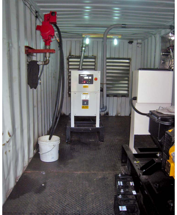
For the new HBS Motor House and Generators, donated and installed by HBS friends in Iowa and Canada, very much needed to be able to carry on our work in Haiti.
