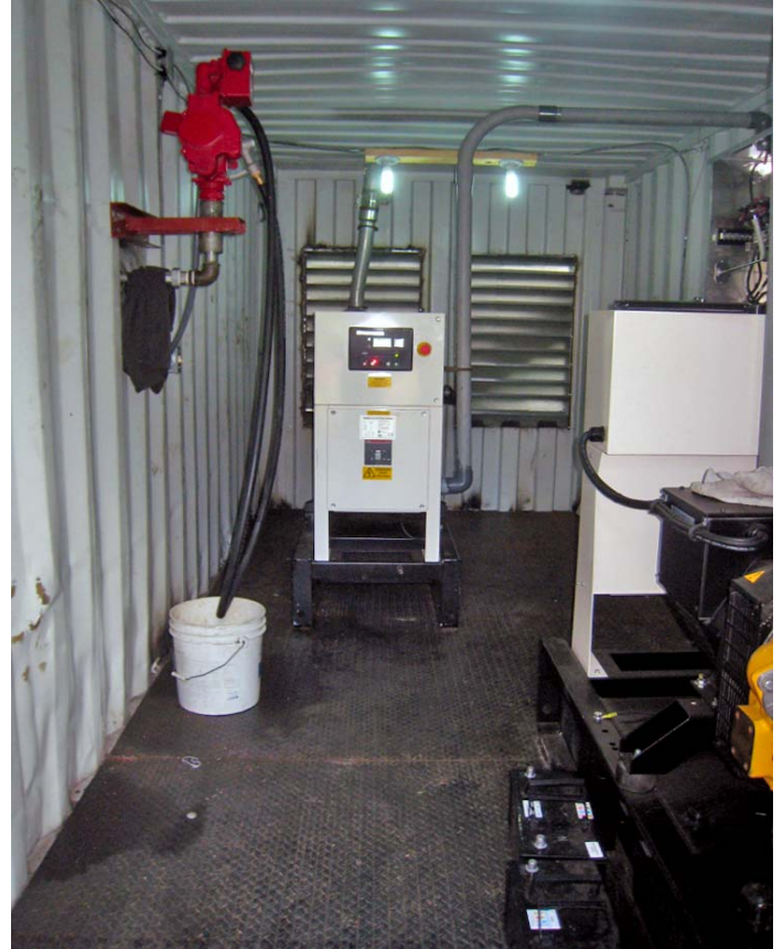
For the new HBS Motor House and Generators, donated and installed by HBS friends in Iowa and Canada, very much needed to be able to carry on our work in Haiti.
