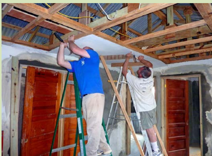
Michael List and Joe Twidwell installing the ceiling for the waiting area in the HIV Clinic.
