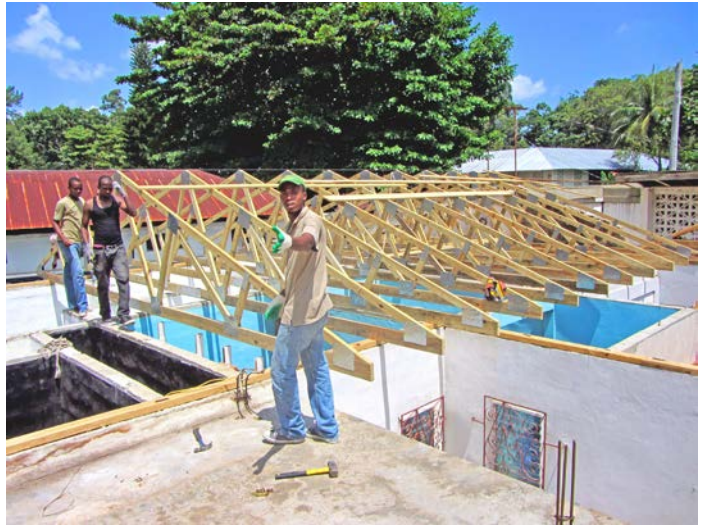
HBS Re-Roofing project is still ongoing. Many of the roofs are over 40 years old requiring replacement of the underlying wood structural supports as well.
