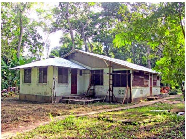
The cafeteria roof has been redesigned and replaced. The work teams arriving in January 2015 will be working on the electrical system and installing a new ceiling.
